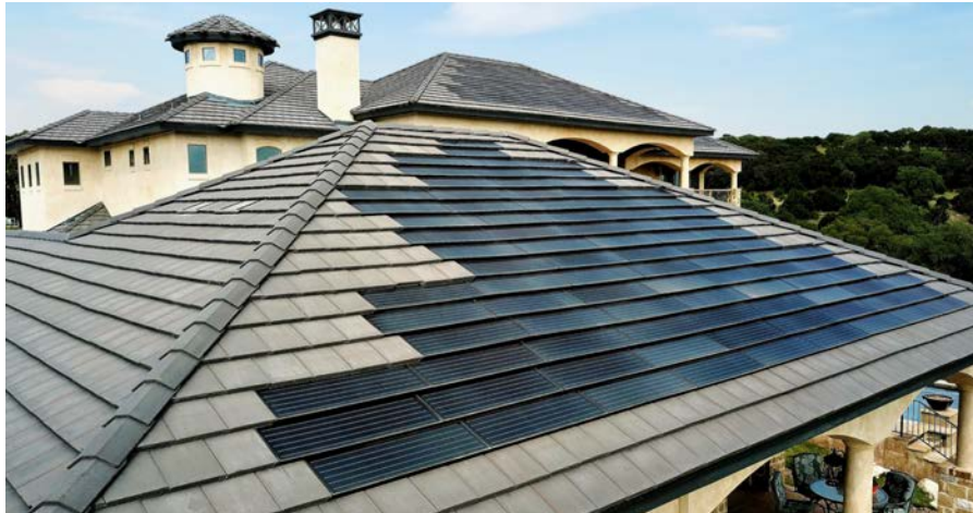
Example above of a "Patchwork" Solar Tile installation that is discouraged.
